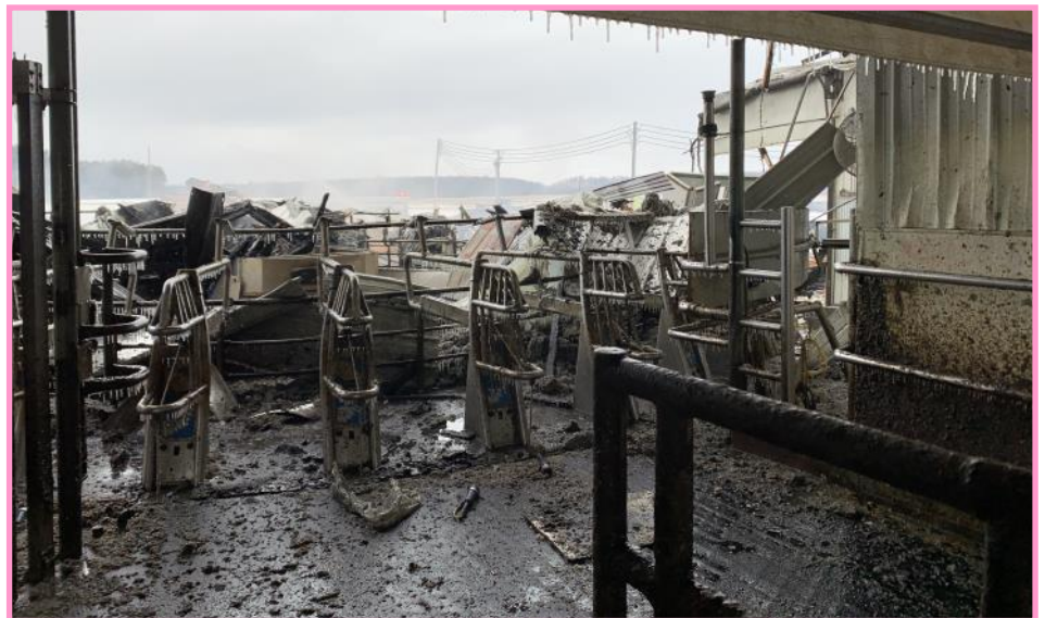
The remains of the parlor milking stalls. (Photo by Hamburg FD.)
